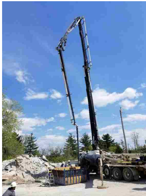
Figure 4-4 Pump on "A" configuration.
